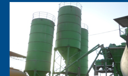
Cement & Fly Ash Silo
